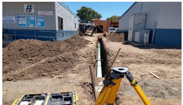
Underground Storm drain
